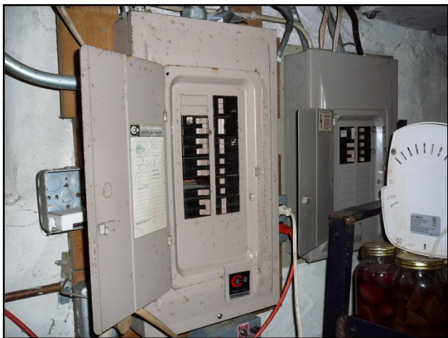
Figure 1- 100 Amp Service Panel
