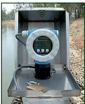
New water level sensor
