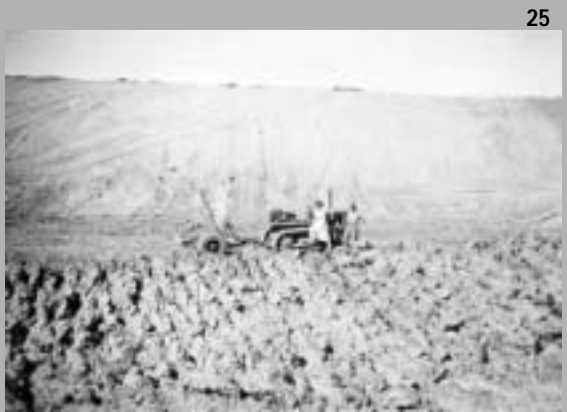
Sinking the main house tank at Mungo with plough and buckscoop using an early model International TD 9 dozer.
