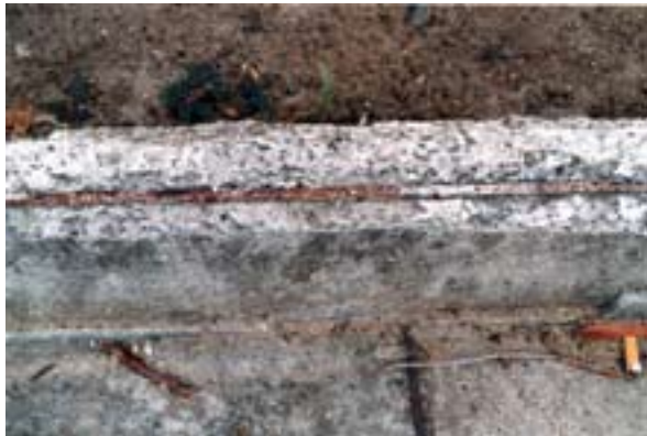
Reinforcing steel exposed and corroding Photo: DIPNR
