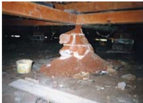
Damage discovered during a building inspection
