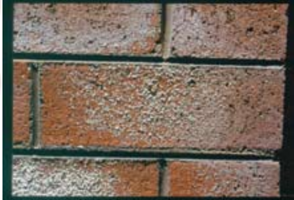
Bricks efflorescing - Photo: NSW Agriculture
