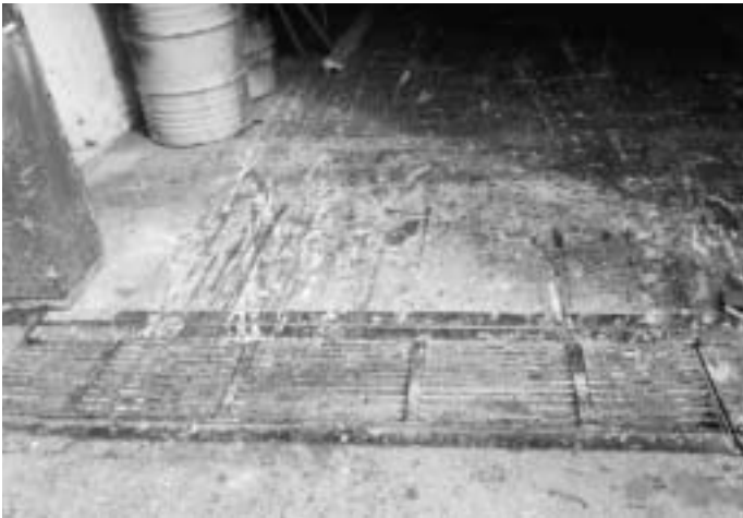
Evidence of paint entering stormwater drain.
