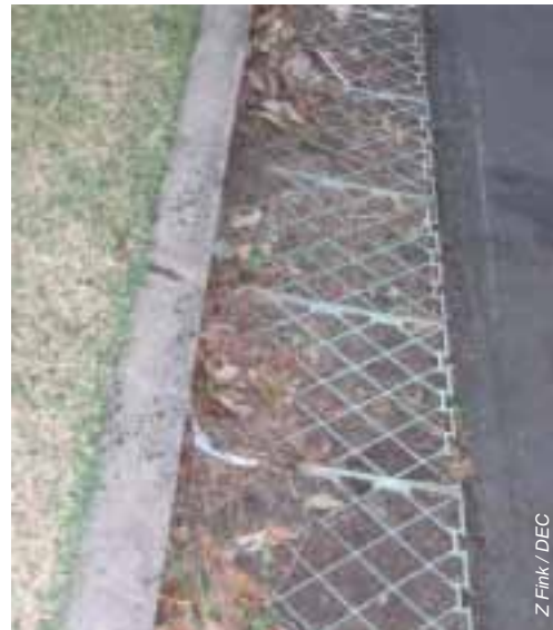
Pervious gutters, North Strathfield (note loss of grass cover in cells)
