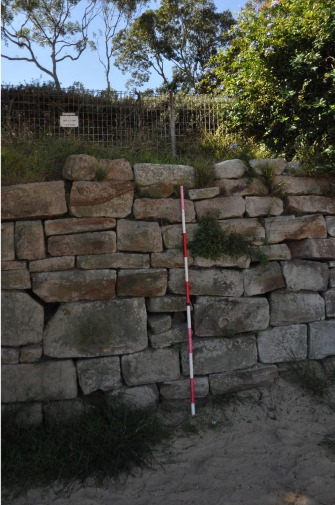
Figure 3.2 View from the beach to the platform on which Constable's Cottage is constructed. The cut and fill process is evident. (Source: GML 2015)
