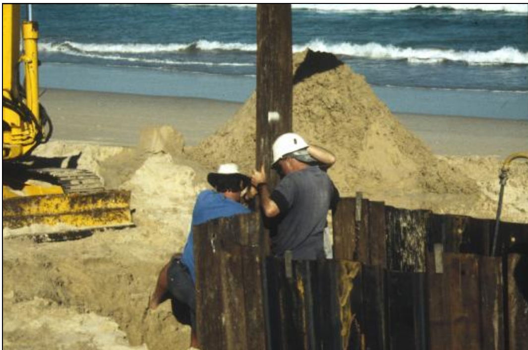
Figure 10: Backhoe removed overburden of sterile sand and drove home the sheet piles.
