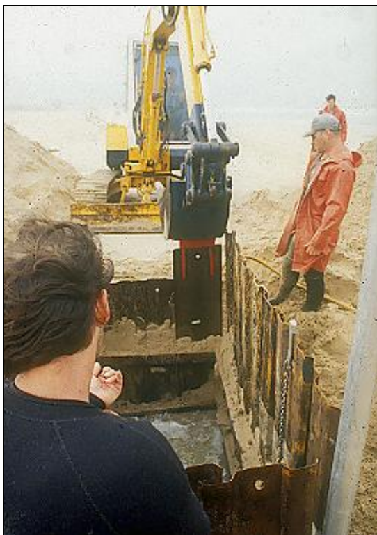
Figure 11: Hydrated sand below the water table moved to refill the excavated caisson, leading to subsidence in the surrounding area.
