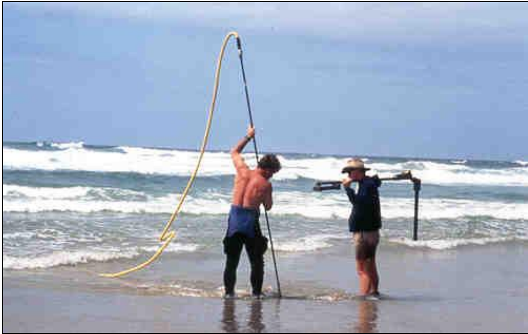
Figure 9: A 4m compressed air probe was used to accurately place the corners of the caisson in relation to the iron object under the sand.
