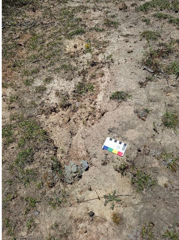
Figure 15: Dispersive light grey slightly humic sandy silts eroding away over more cohesive sub-soil clays and clay silts. Scale intervals 1cm on black and white squares.
