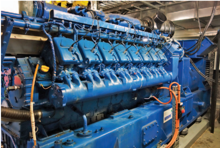
Figure 35: Gas-fired reciprocating engine and generator
