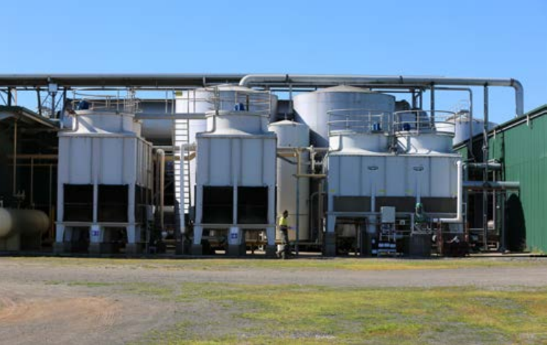
De Bortoli Wines' refrigeration system cooling towers
