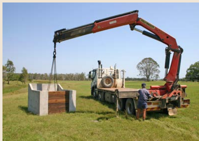
A new water control structure during the installation process. Landholders now use these structures to regulate water levels
