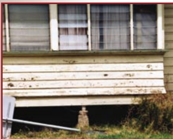
Salt and water damage to a pier. Photo: DIPNR
