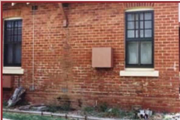
Salt and water impacts exacerbated by a disconnected downpipe.
