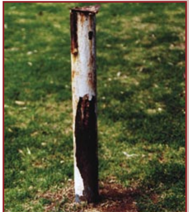
Rusted piezometer. Photo: DIPNR
