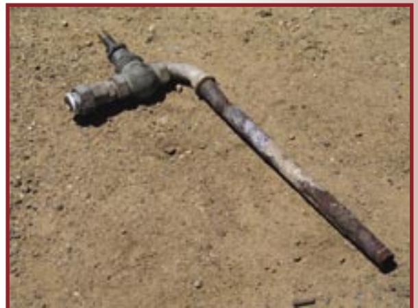
Rusted pipe. Photo: NSW Department of Primary Industries
