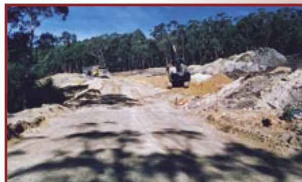
Road construction can change natural drainage patterns. Photo: DIPNR
