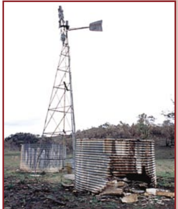
Rusted water tank. Photo: NSW Department of Primary Industries
