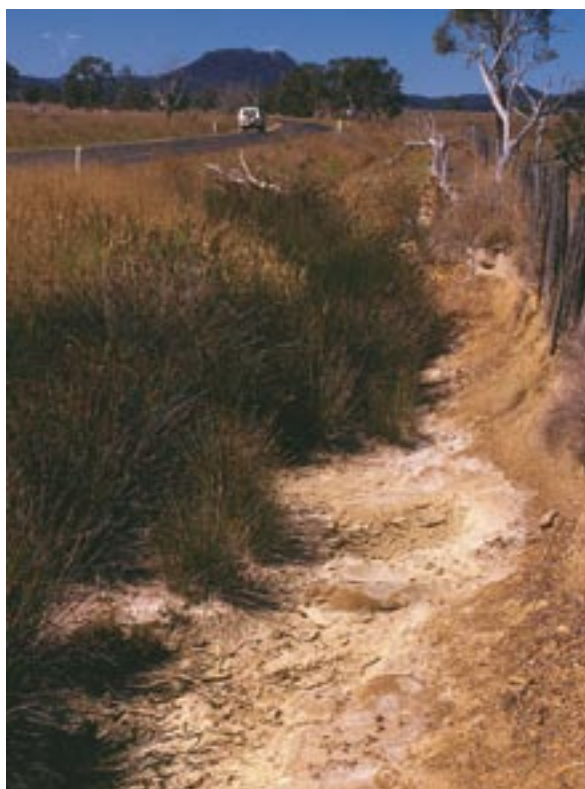
Salt accumulation in a road culvert. Photo: Department of Primary Industries
