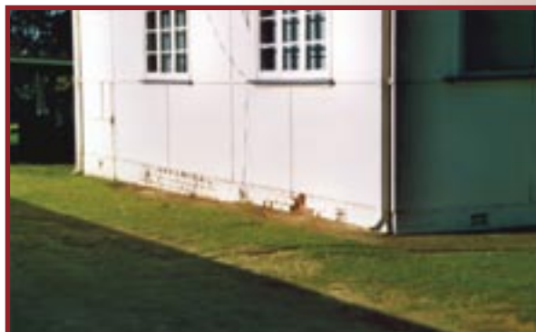
The impact of salt and water on brickwork. Photo: DIPNR
