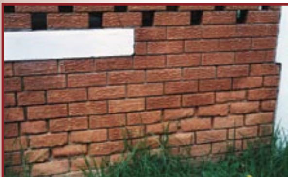
Bricks showing signs of salt and water impacts. Photo: DIPNR
