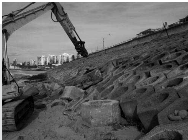
The Prince Street seawall at Bate Bay is being upgraded to protect the bay's foreshore.
