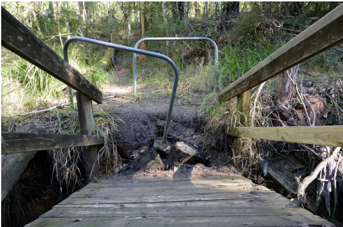
Photo 2: Damaged bridge section
