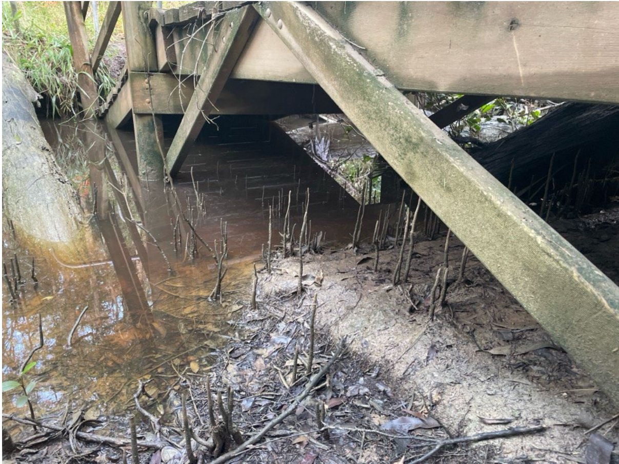
Photo 2 Example of the current condition of the bridge within the tidal channel
