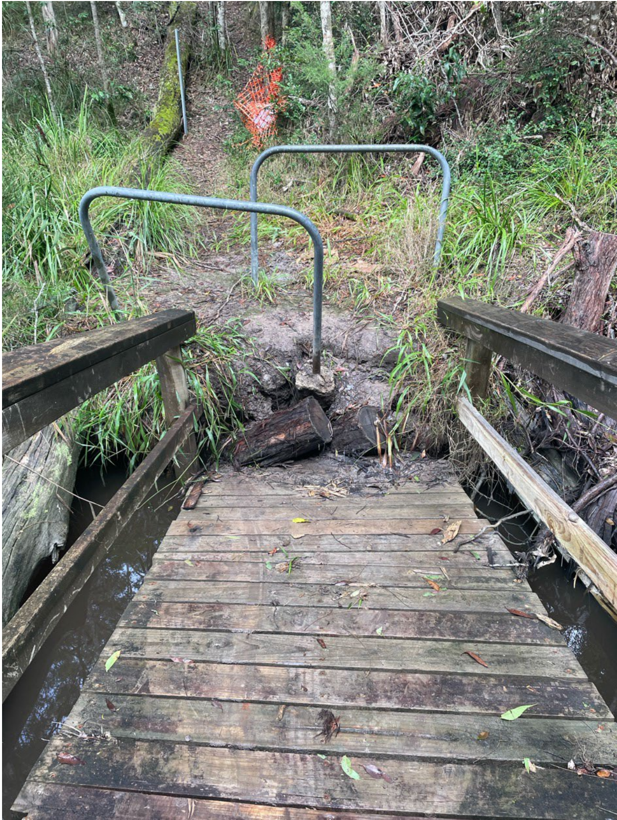
Photo 1 Collapsed bank and bridge failure
