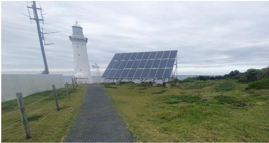
Photo 6-5: NPWS off grid power supply
