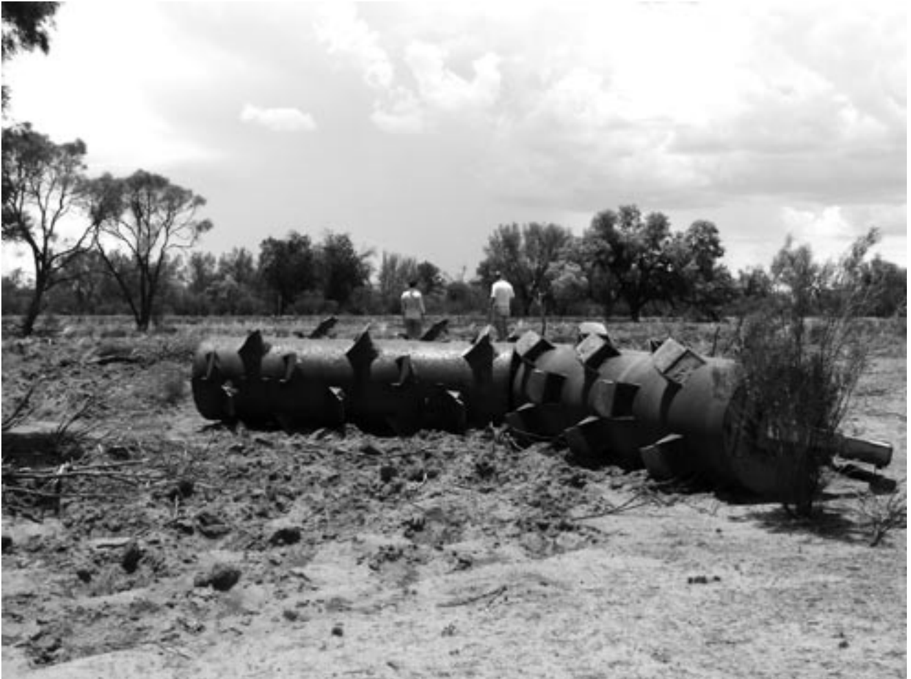
Using a 'crocodile' to control invasive native scrub near Fords Bridge in western New South Wales
