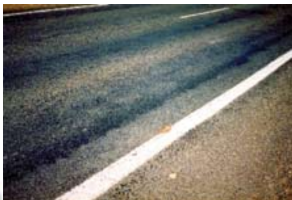
A highway with blistering of the seal
