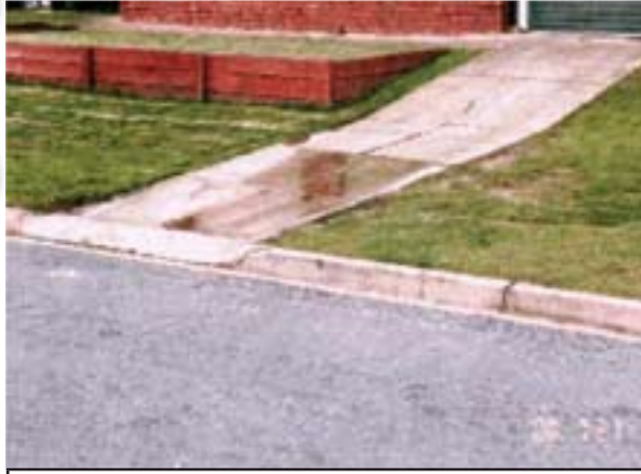
An urban driveway with groundwater seepage
