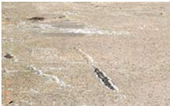
Water & salt crystals in cracks in a carpark
