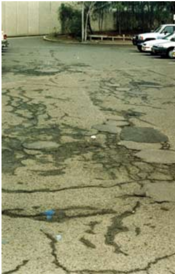
Carpark showing damage
