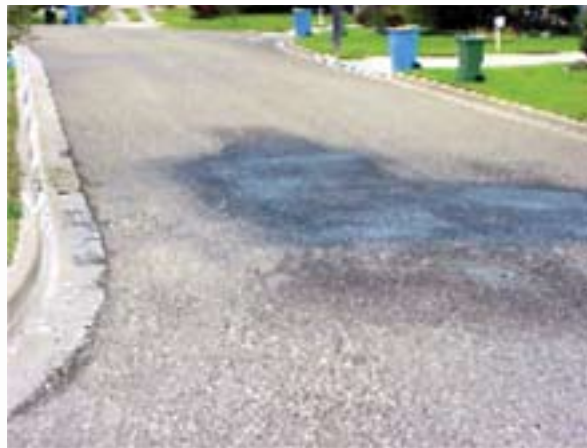
An urban road showing damage
