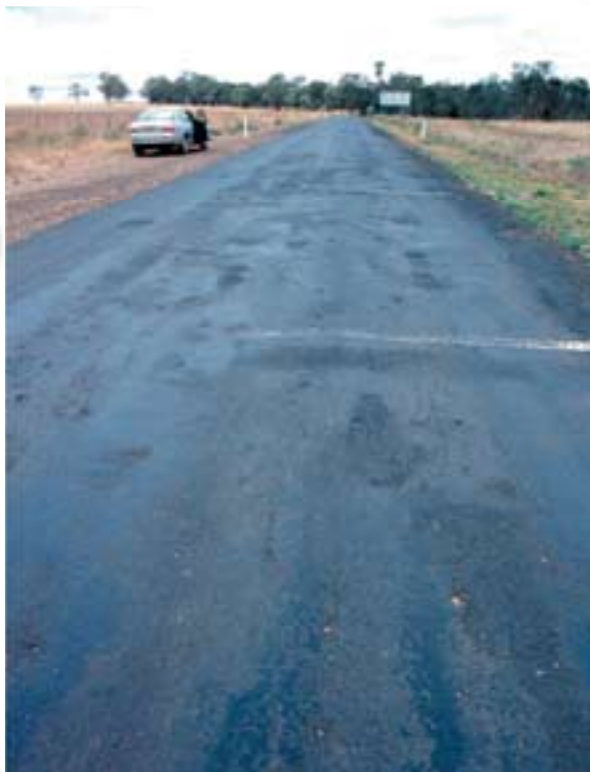
A rural road showing damage
