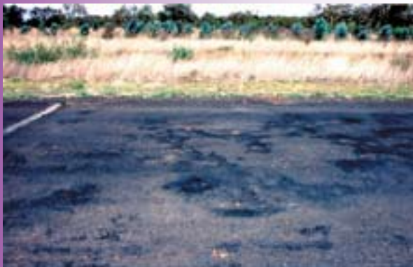
Numerous blisters in the seal of a rural road
