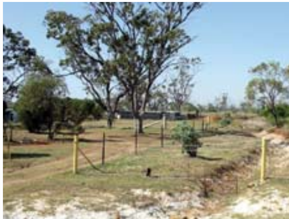
A rural stormwater drain showing salinity symptoms
