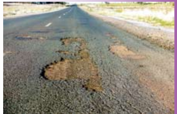
A rural road showing damage
