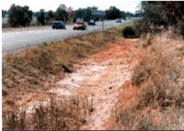
A roadside drain with visible salt crystals
