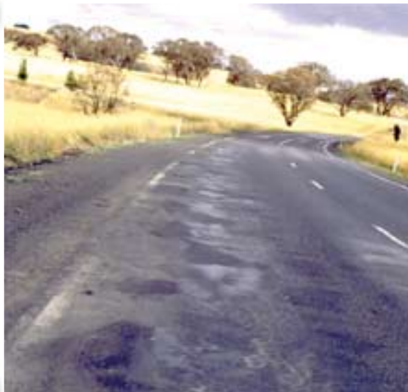
A rural road with “deformation”
