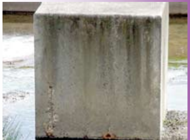
Exposed reinforcing in a concrete piling
