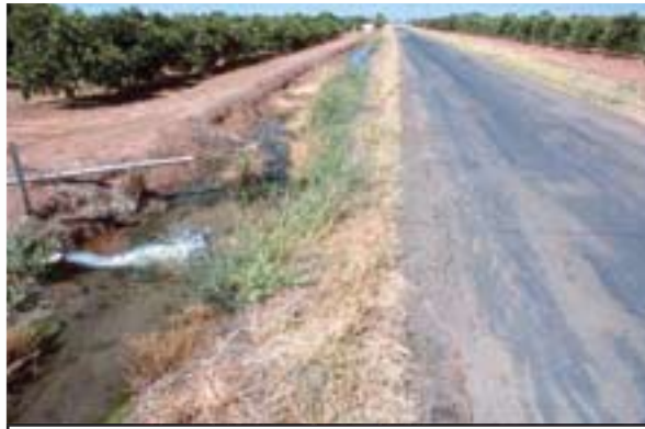
A road in an irrigation area showing damage
