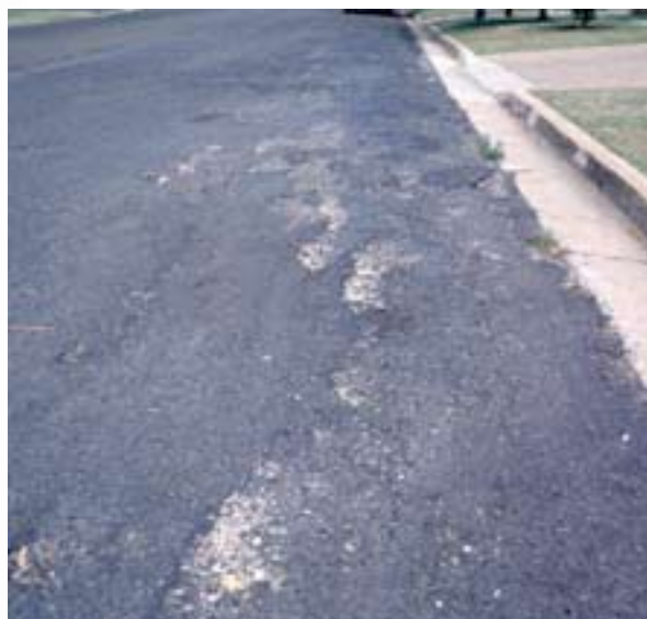
An urban road showing damage
