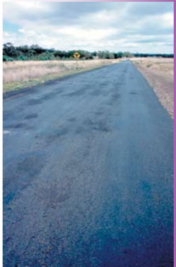
A rural road showing damage
