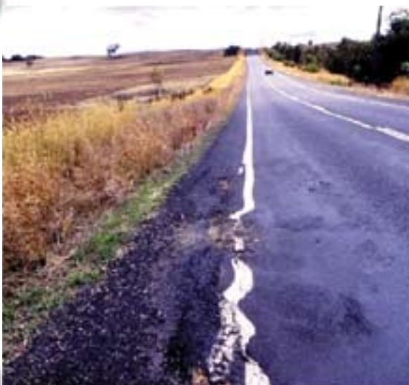
Deformation of a rural road
