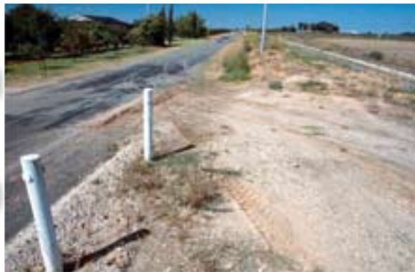
A rural road showing damage
