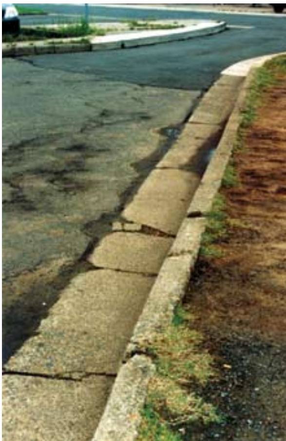
Gutter, road and nature strip with salinity damage
