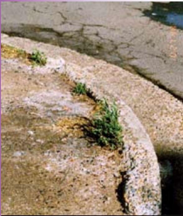
Kerb and guttering affected by sulphate salts
