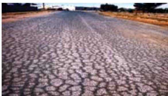
Cracking of a road exposed to high levels of moisture
