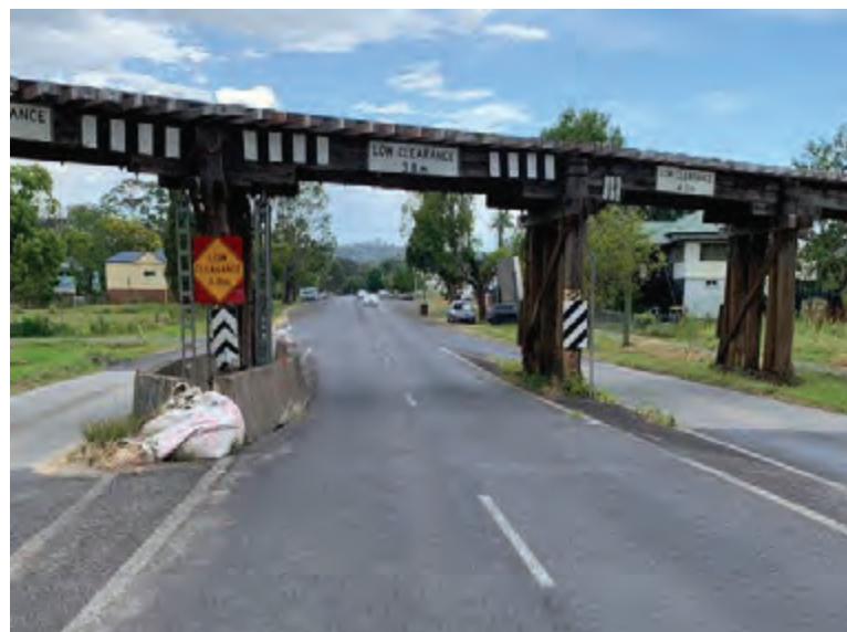
Photo 8: Narrow road width centre span - Terania Street viaduct
