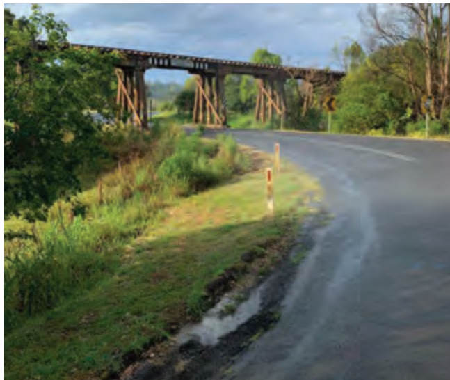
Photo 20: Roadside hazards – embankment on inside of bend (northbound) – Winterton Parade
