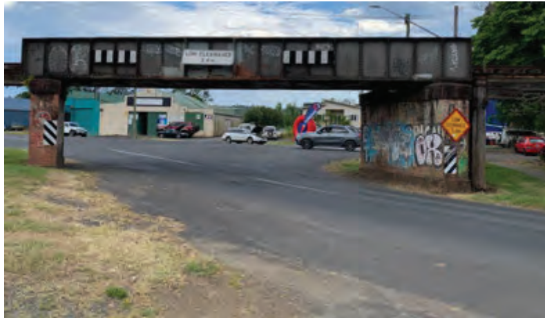
Photo 1: No edge lines - Union Street viaduct
