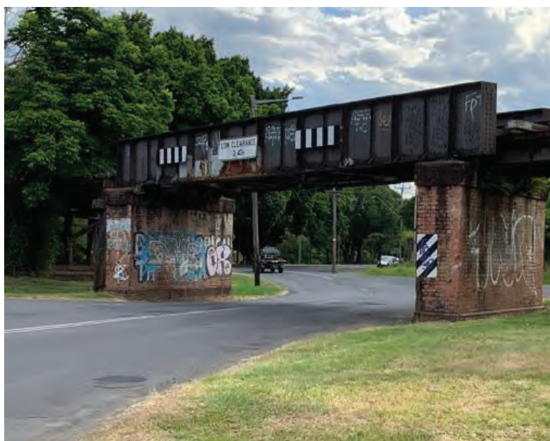
Photo 3: Missing width marker on pylon - Union Street viaduct
