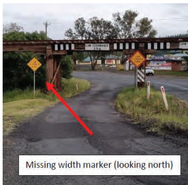
Photo 27: Missing width marker – Winterton Parade viaduct eastbound
