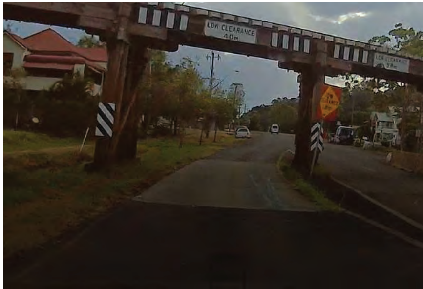
Photo 10: Minimal edge clearance - Terania Street viaduct
