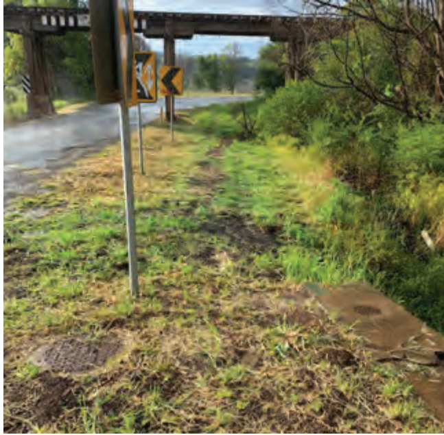
Photo 19: Roadside hazards – drain and trees on outside of bend (northbound) – Winterton Parade
