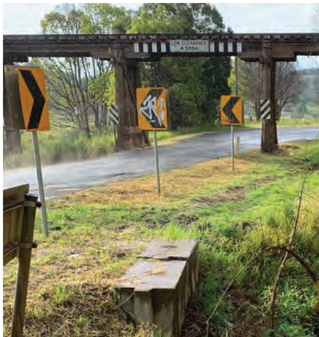
Photo 23: Vandalised signs – Winterton Parade viaduct
