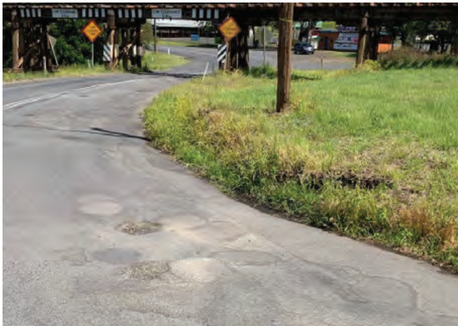
Photo 32: Lack of roadside drainage – Alexandra Parade eastbound, south of viaduct
