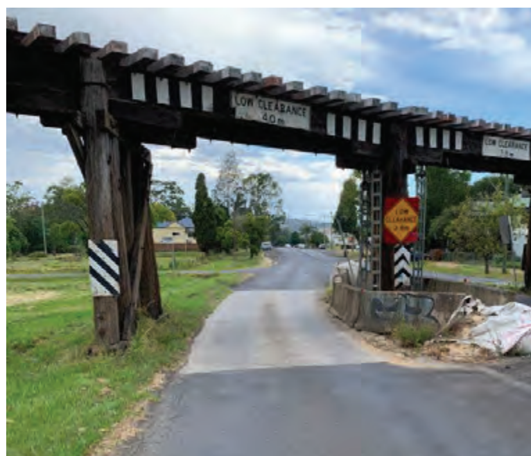
Photo 9: No edge lines - Terania Street viaduct
