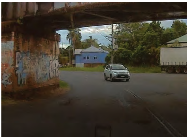
Photo 2: Minimal edge clearance - Union Street viaduct
