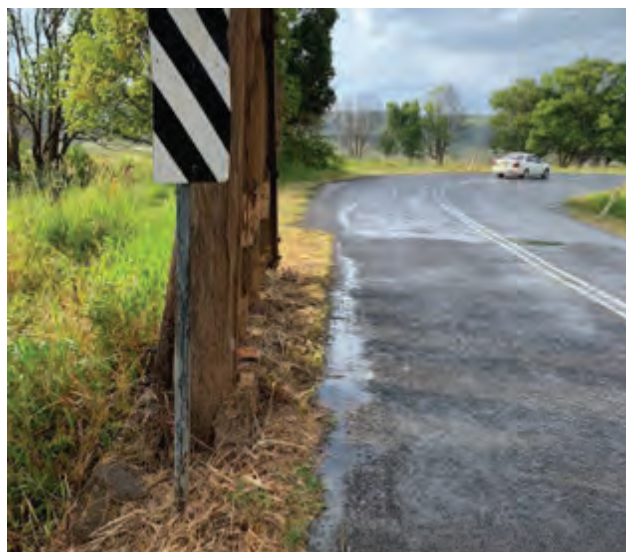
Photo 15: No edge lines and minimal edge clearance - Winterton Parade viaduct
