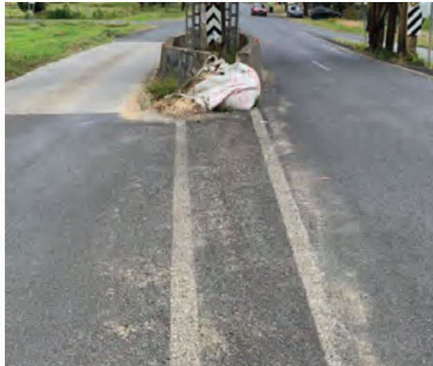
Photo 14: Poor condition and placement of lines - Terania Street viaduct
