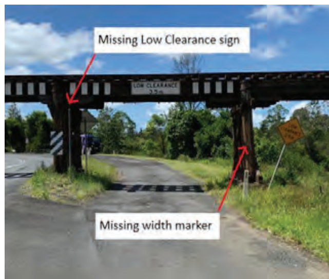
Photo 26: Missing width marker and Low Clearance sign – Winterton Parade viaduct eastbound
