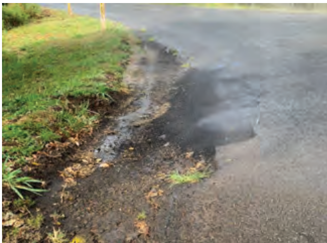
Photo 21: Damaged road pavement - inside of bend (northbound) – Winterton Parade
