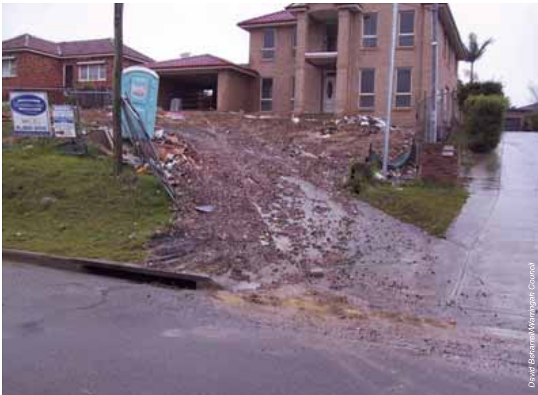
Badly managed construction sites are all too common
