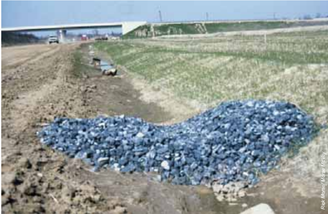
An effective check dam traps sediment by slowing flows
