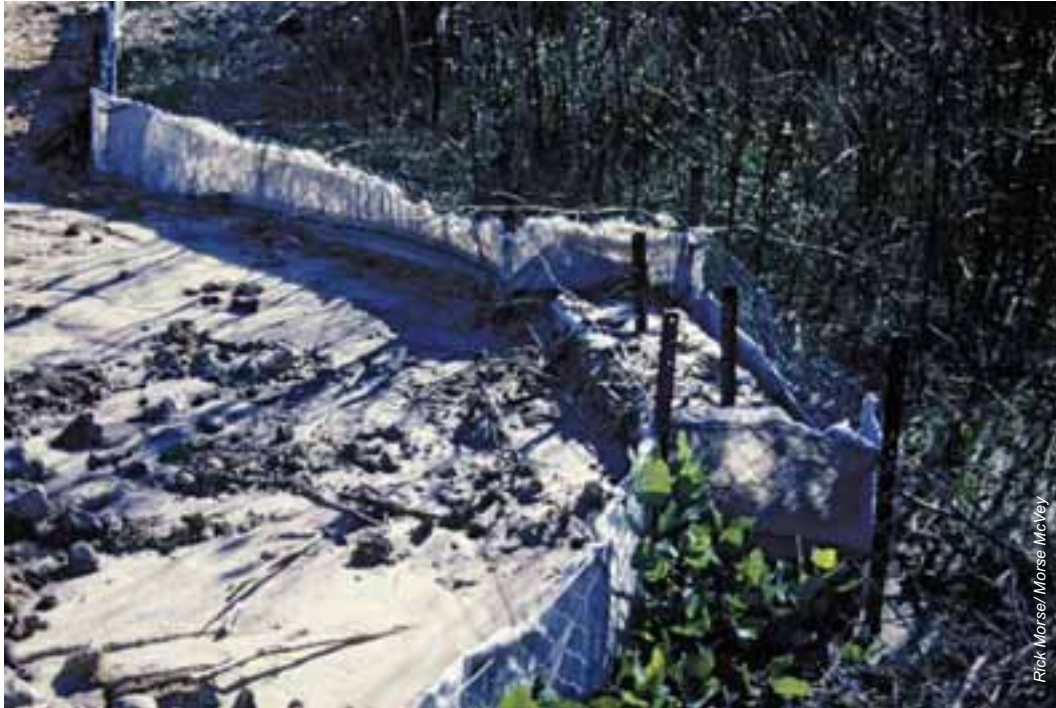
A simple but effective sediment trap made with fencing and straw bales
