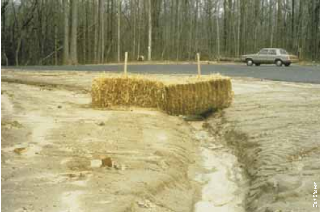
Poorly installed straw bales
