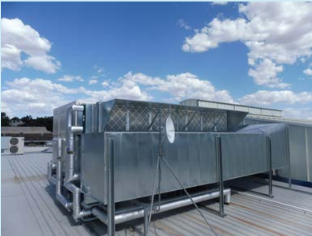
Figure 3 Exchange ventilator unit with LPHW (ESBS Pty Ltd)
