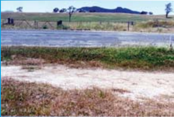
Salinity indicators at this site include road damage, sea barley grass, bare soil and salt crystals. Photo: NSW DPI
