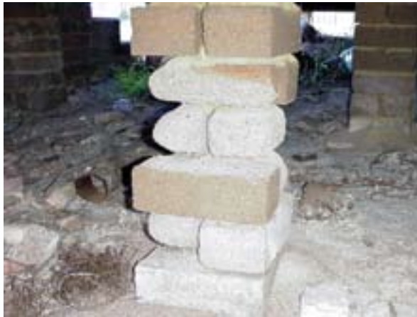
Salinity may cause structural damage to bricks and mortar. Photo: DNR
