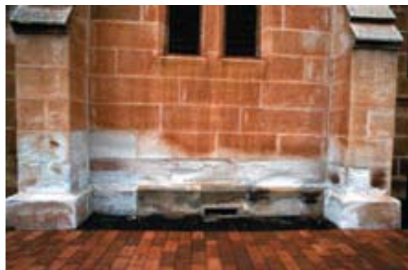
Heritage buildings can also be affected by salinity. Photo: NSW DPI
