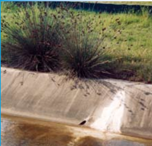
Salinity indicators at this site include white salt crystals, unexplained water seepage, clear water and salt tolerant plant species. Photo: DNR
