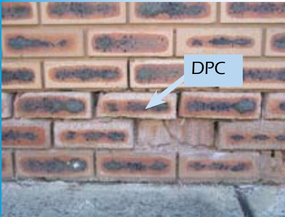
Salinity damage is minimised to the area below the damp proof course (DPC) in this building. Photo: Campbelltown Council
