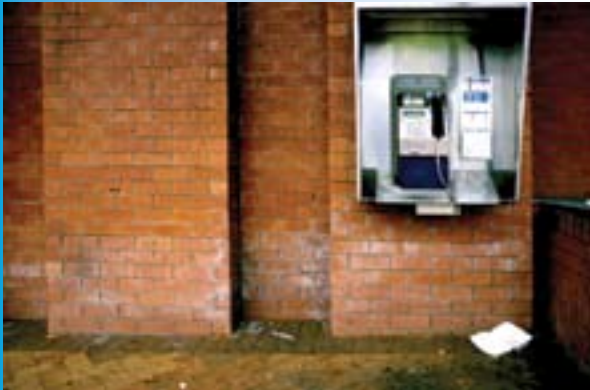
Efflorescence on the wall of a public building. Photo: NSW DPI
