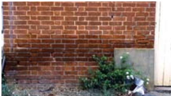
Tide mark on wall indicating the presence of water. This could be groundwater close to the surface or a leaking pipe. Photo: NSW DPI.
