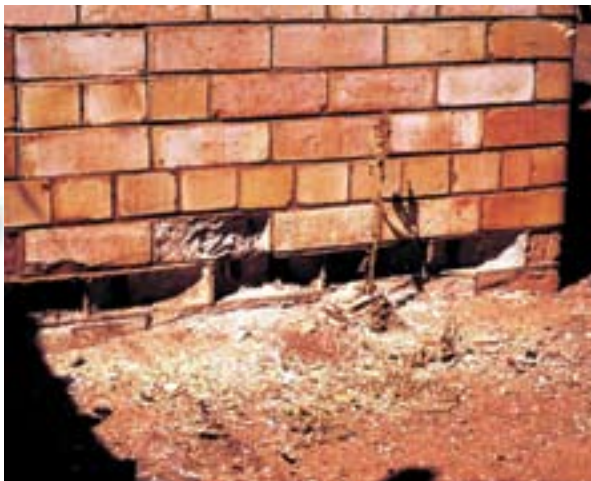
Damage to bricks and mortar caused by salinity. Photo: NSW DPI.
