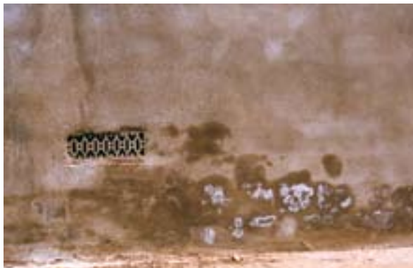
Render showing signs that excess water and salt are present. Photo: NSW DPI
