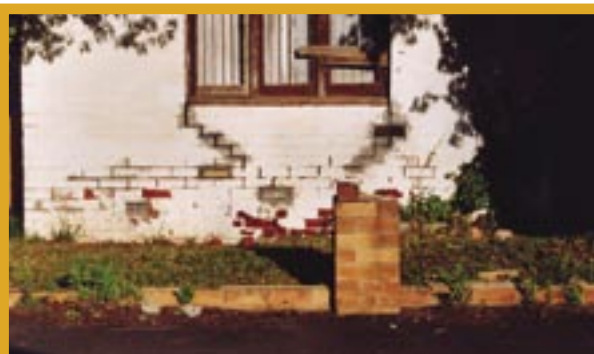
Salt and water have affected the paintwork and mortar on this property. Exposure class bricks and mortar are more resistant to the impacts of salinity.
