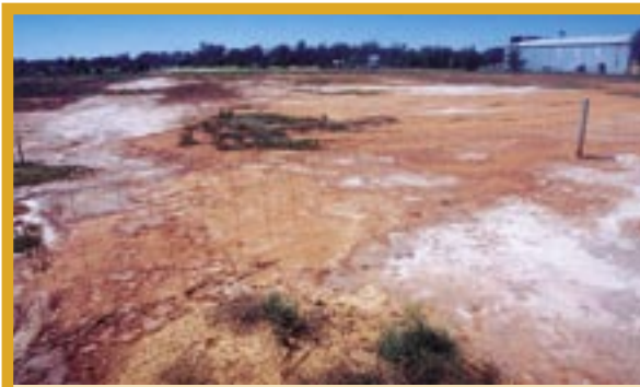
This undeveloped property in an industrial estate has salt crystals on the soil surface. These are only visible when rain, dew and other forms of moisture are insufficient for the salt to be dissolved.
