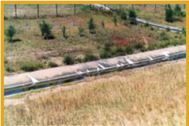
Salinity indicator plants, salt crystals, groundwater seepage and poor soil structure are evident in this stormwater easement through an industrial area. Tree planting will help lessen the impacts of salinity processes while providing other benefits such as habitat.
