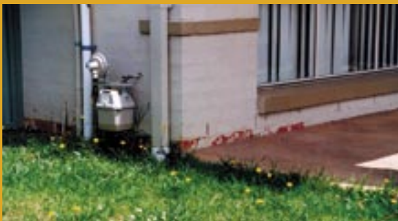
Salinity indicators such as flaking paint, mortar, render and bricks may be evident on old and new houses. Some may be caused by other factors such as a leaking pipe.
