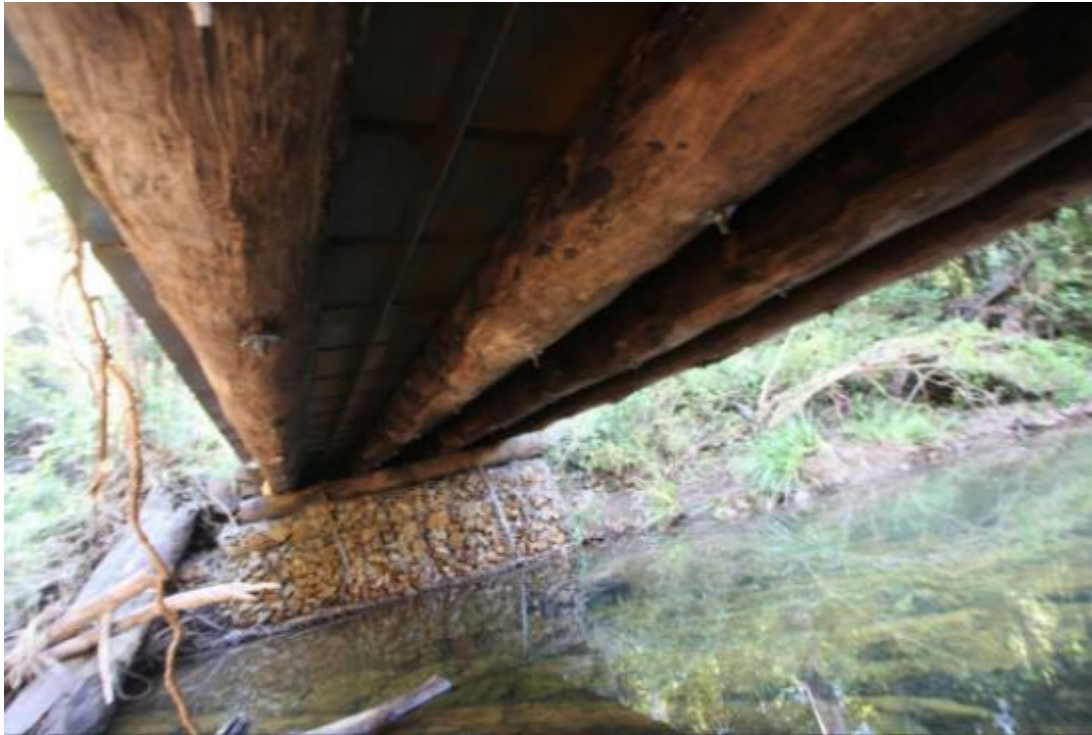
Figure 7 Buds Crossing Road Bridge deck girders and underside of the concrete deck, facing north (Everick 2021b)
