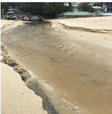
Stormwater drain flow Photo: Beachwatch/DPE
