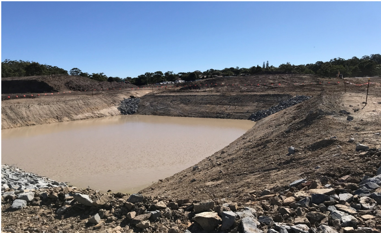
Type D Basin. Photo: Design Flow Consulting
