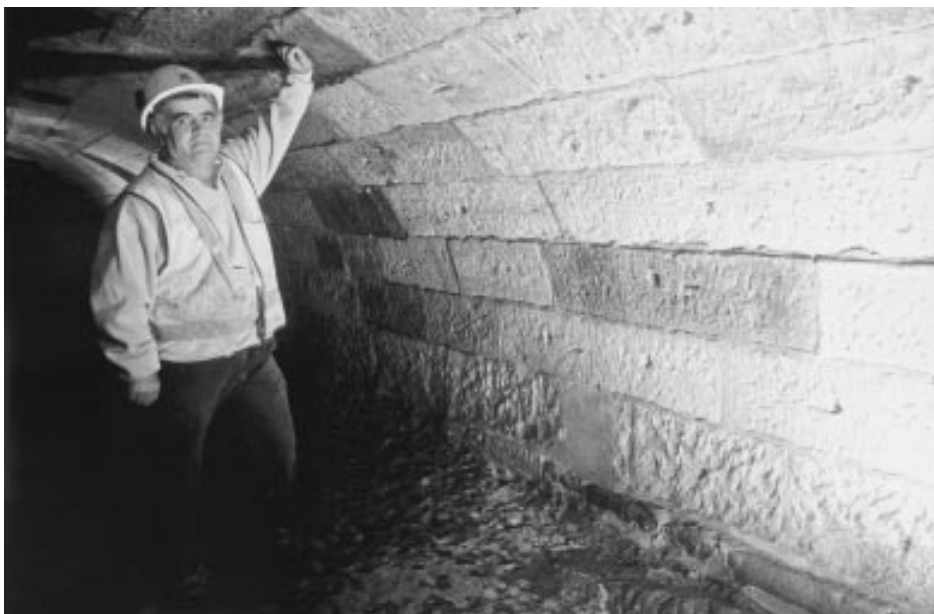
Water Services Officer Leo Geraskis in the Tank Stream, the watercourse that supplied the early colony of Sydney with fresh water. This year Sydney Water celebrated the listing of nearly 30 of its most significant assets on the State Heritage Register. Photograph by Neil Holbrook, courtesy of Sydney Water Corporation
