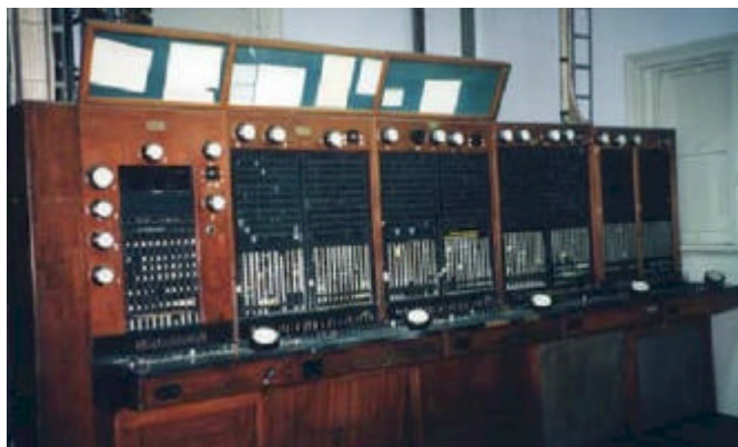
Early telephone exchange with heritage significance
