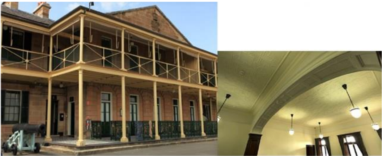
Officers' Quarters, Paddington Barracks, Paddington: These historically significant pressed metal ceilings were restored using intumescent paint that gave FRL of 90/90/90.
