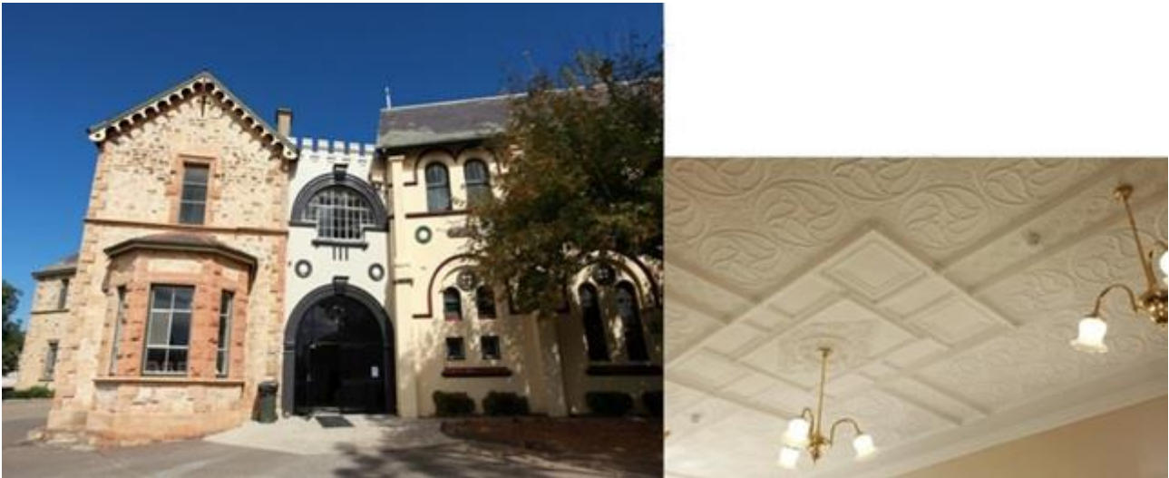
Trinity College, Goulburn: Intumescent paint used to achieve FRL of 90/90/90 while preserving ornate fibrous plaster ceiling (lath and plaster substrate) and pressed metal ceiling.
